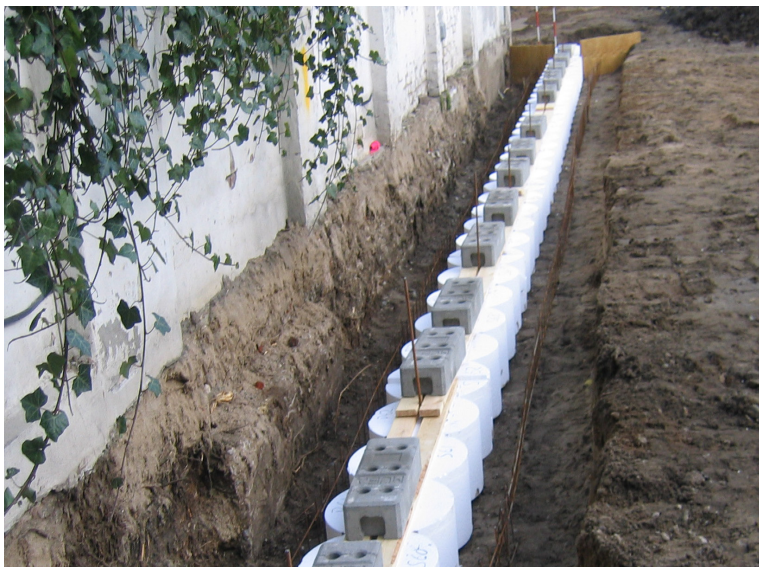
The work starts with construction of a guide wall, so that the centre distance between the piles corresponds exactly to the required overlap.
