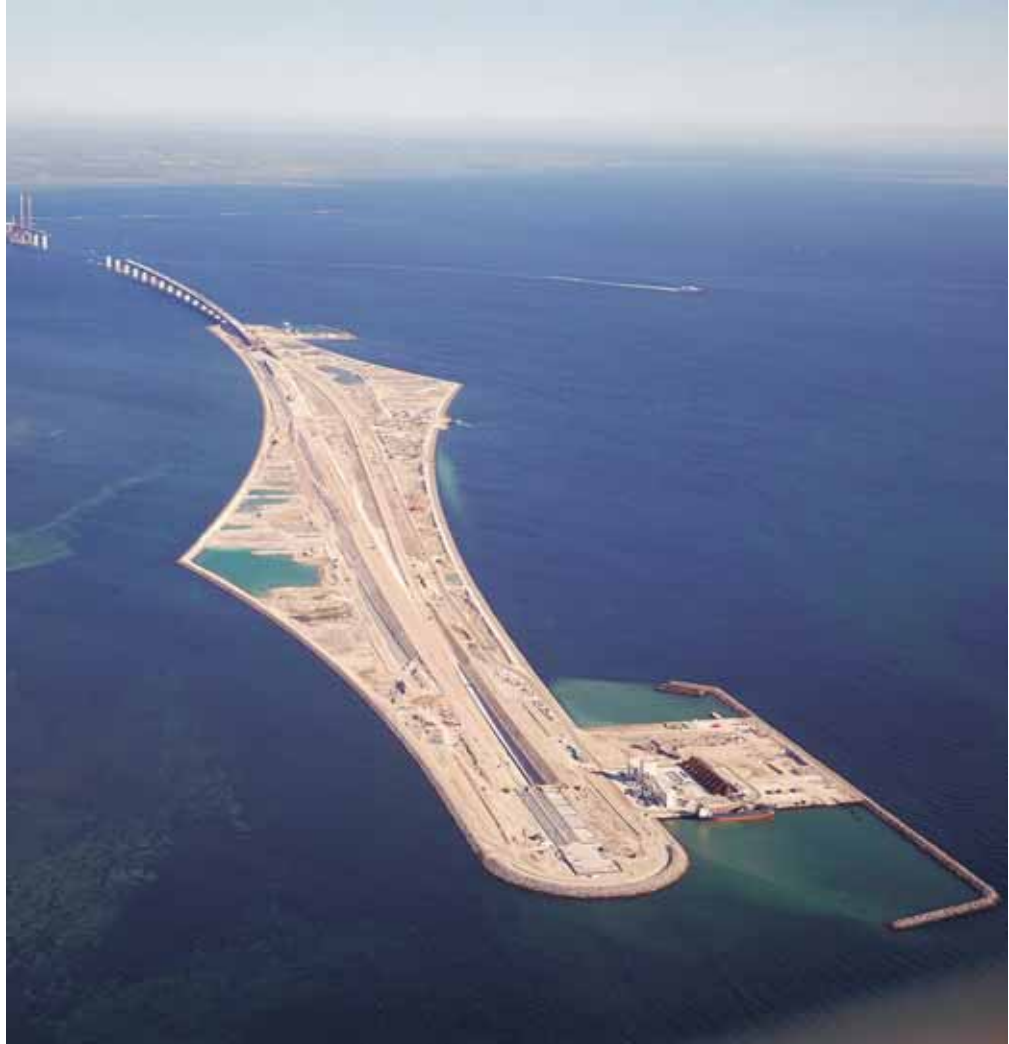
Looking East across the island towards Sweden. The motorway seen on the left, and railway, on the right, are taking final form.
