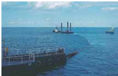
Side-wire system in place for the "Castor".
