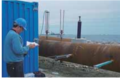
Weir Box Station located on the artificial island.
